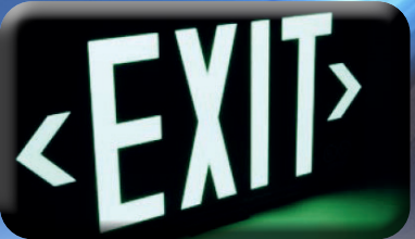
Security System & Emergency Lighting
