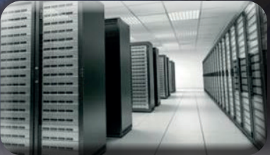
UPS & Data Centre
