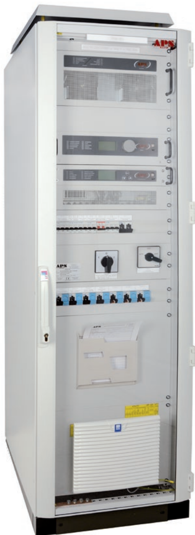
PIC. FAT in industrial cabinet
